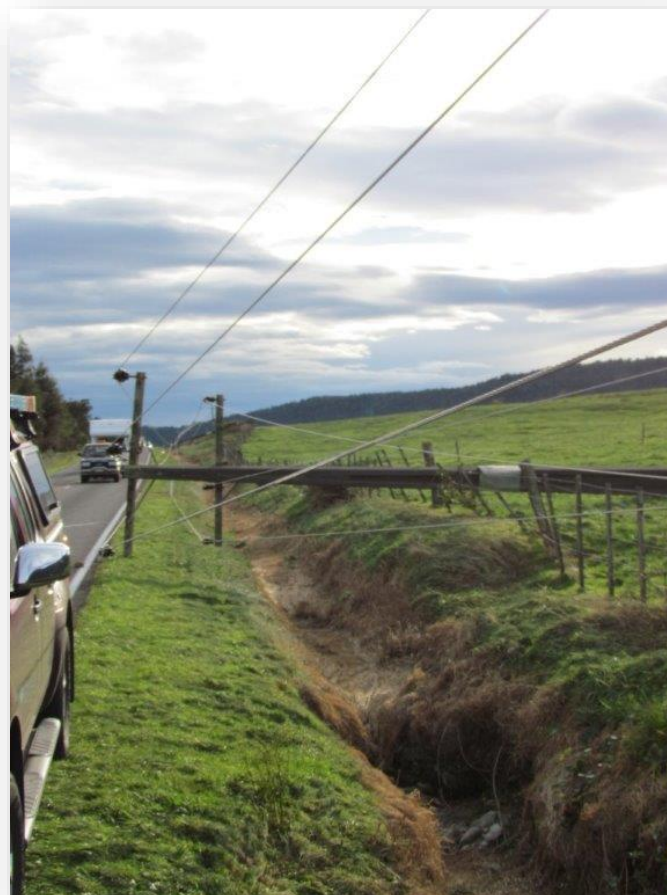
Damaged powerlines, South Westland.
