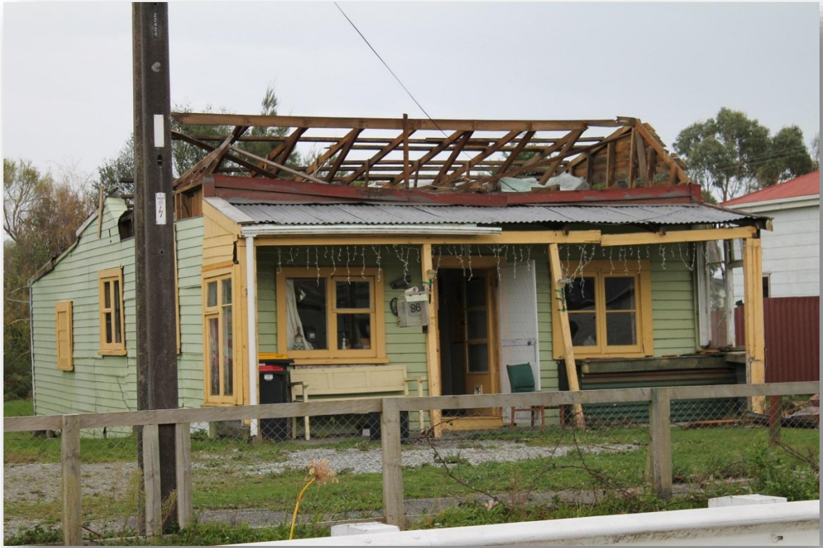
Damaged Cobden house. Photo courtesy of the Greymouth Star
