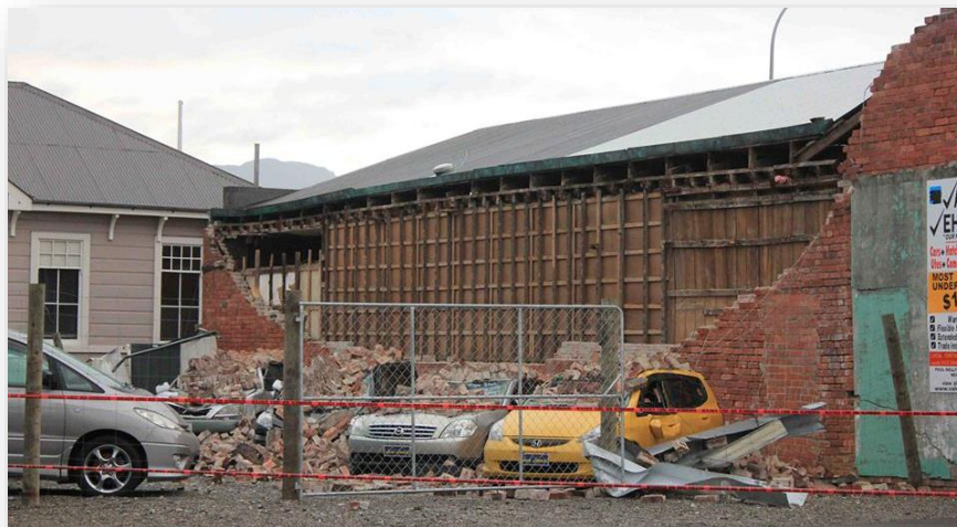
Collapsed brick wall, Westport.
