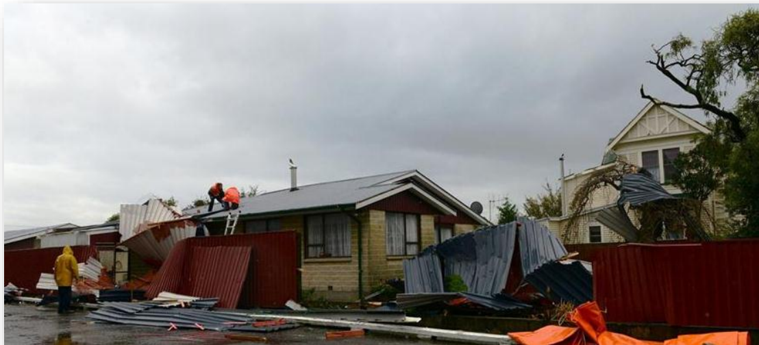
Damaged properties, Westport. Photo courtesy of the New Zealand Transport Agency
