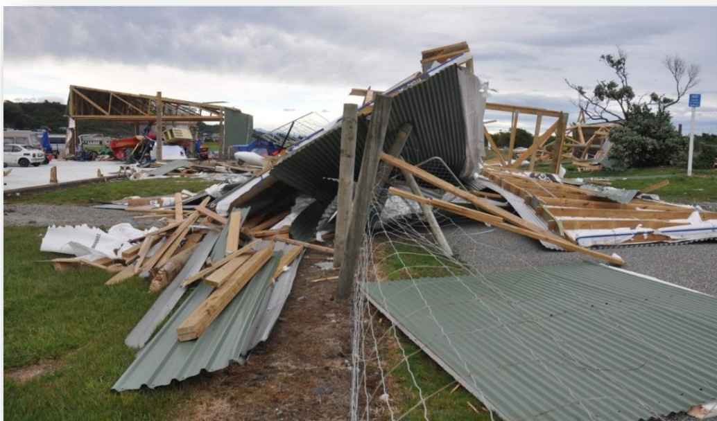
Damaged Greymouth Aerodrome Hanger. Photo courtesy of the Greymouth Star
