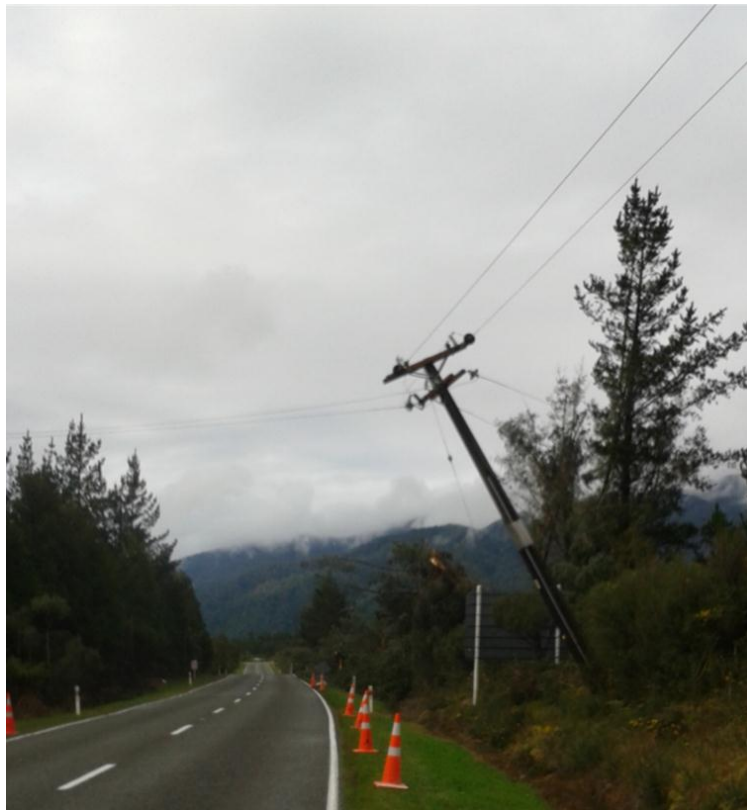
Power poles and lines damaged, Buller District.
