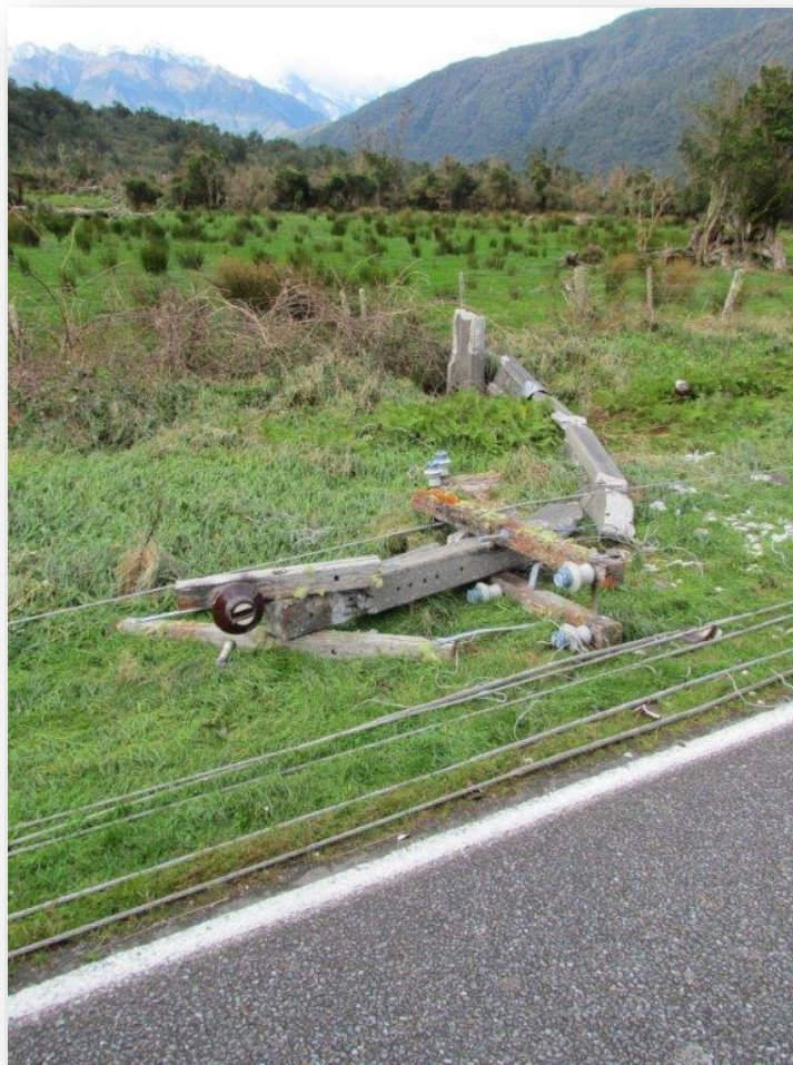
Disintegrated powerpole, South Westland.
