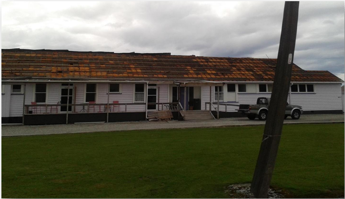
Roof damage to the Whataroa Motel.
