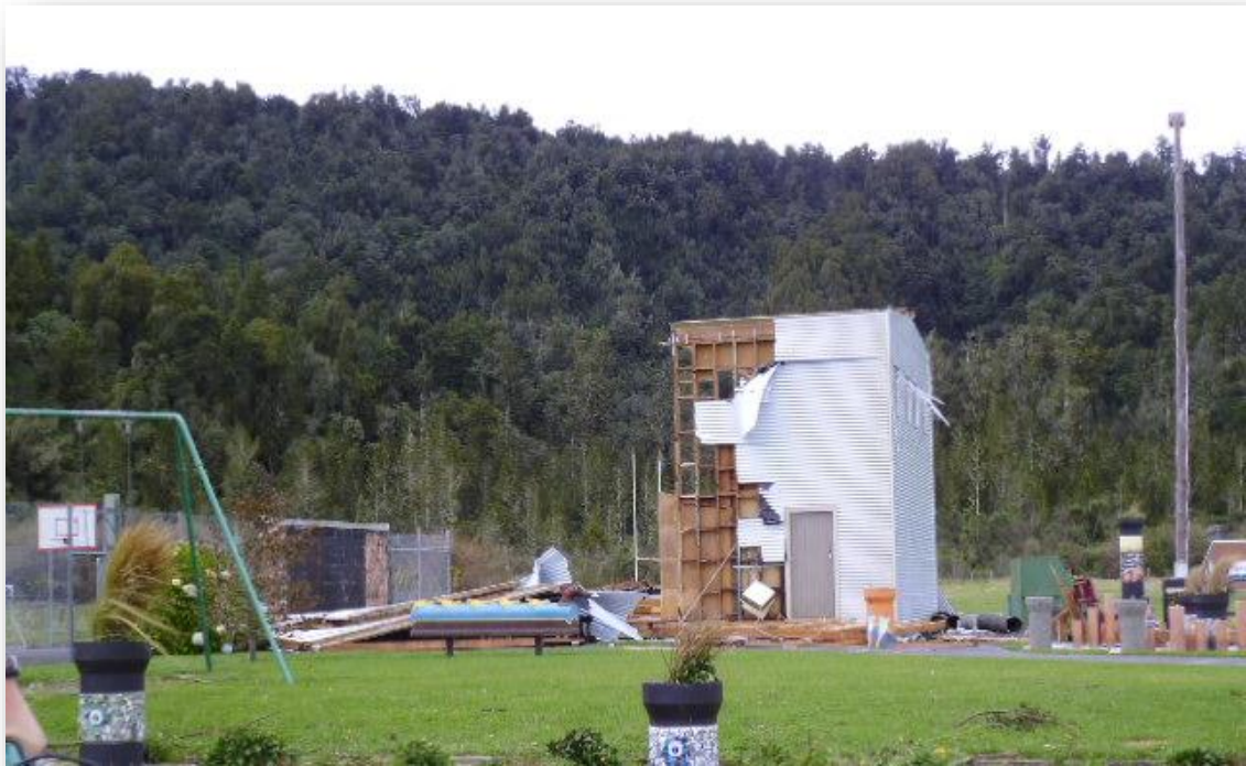
Damage to Harihari squash courts. Photo courtesy of Westland District Council
