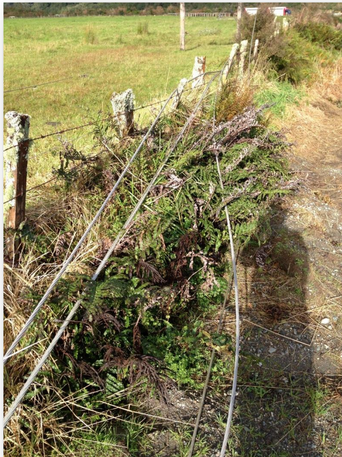
11000 volt power wires across a farmers fence.
